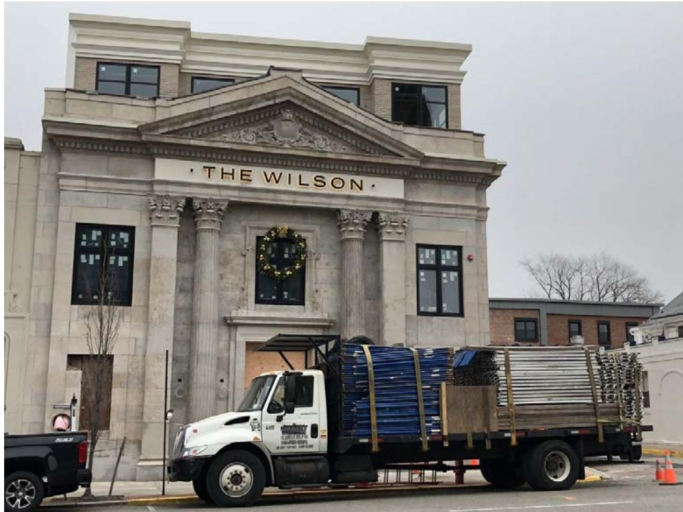
The scaffolding is removed from The Wilson building on Bloomfield Avenue in Caldwell on Monday, Dec. 9.
